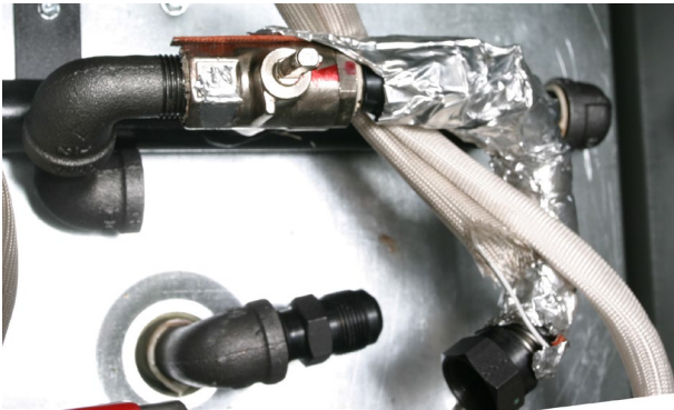
Figure 3: The front flush hose is shown disconnected.
