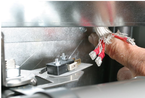
Figure 1: The wires are shown removed from the drain microswitch.
